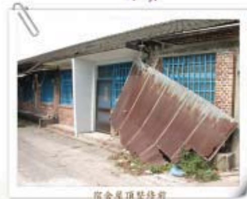
宿舍屋頂整修前
